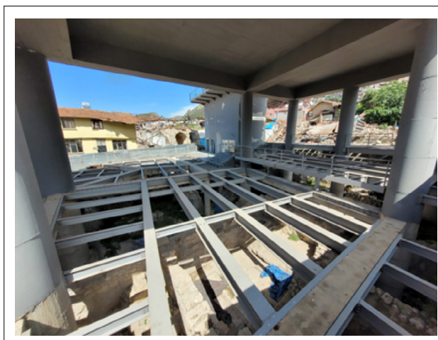
Figure 22. General view of the site after the earthquake.
