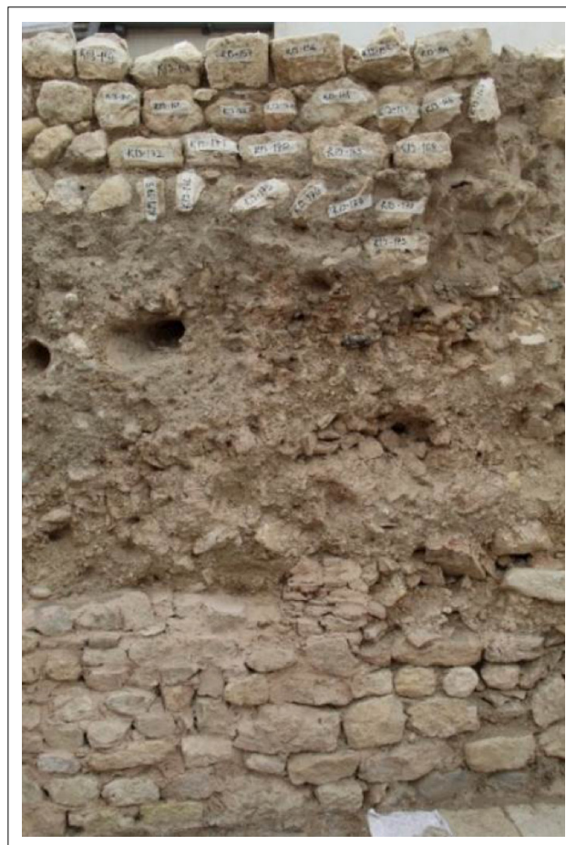
Figure 12. Weak masses containing soil, rubble, and broken terracotta fragments that are prone to erosion by rain.
