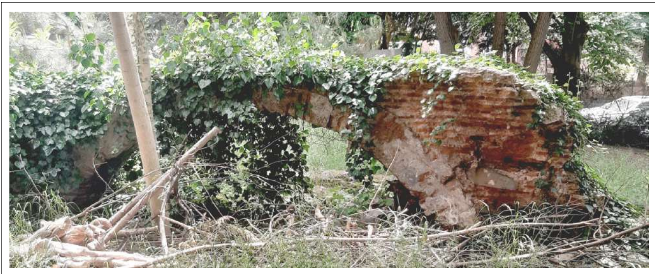
Figure 6. Arched wall element observed during the exploratory filed survey.
