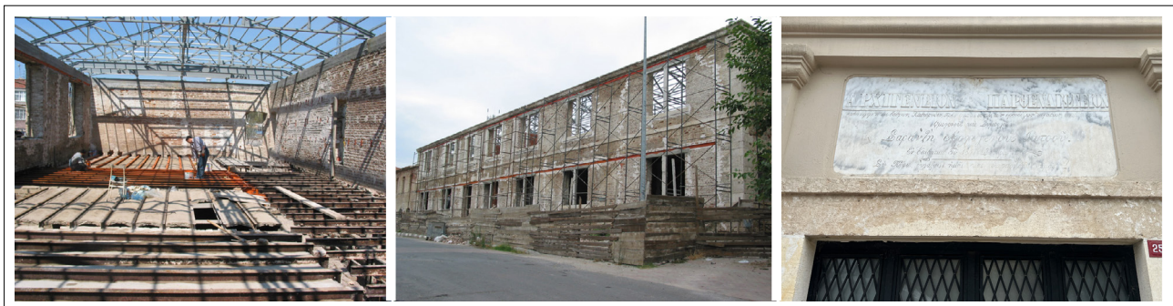
Figure 12. Reconstruction of the roof and floor systems during the repair of Block 2, consolidation of the brick walls, and the present state of the conserved marble inscription (Hanart Architecture Archive).
