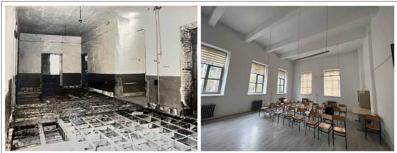
Figure 19. Dismantled wooden slab of the upper floor (Conservation Council Archive), Interior was reconstructed using reinforced concrete.
